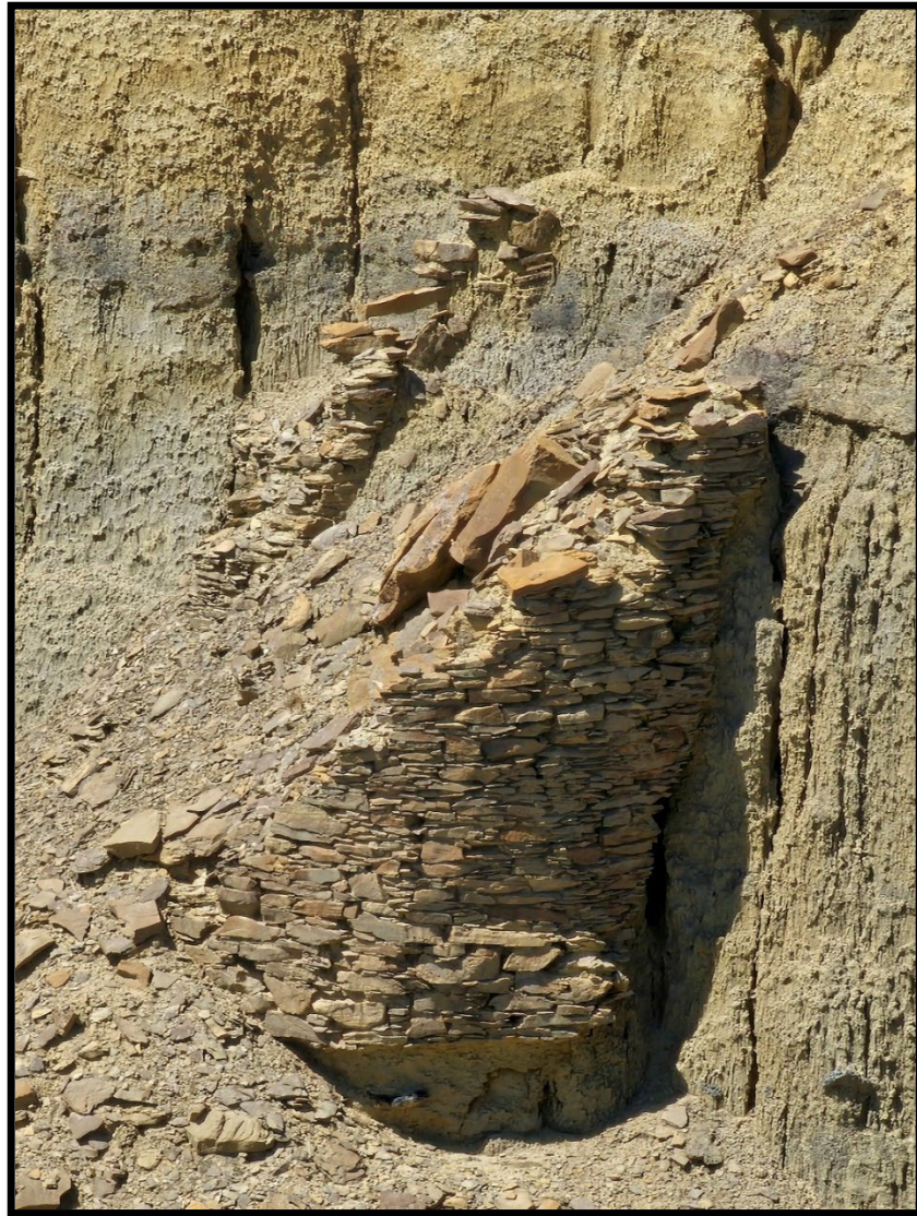
Figure 7: Masonry structure under threat from erosion
